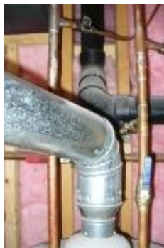
Photo 68 Main interior shut offs.
