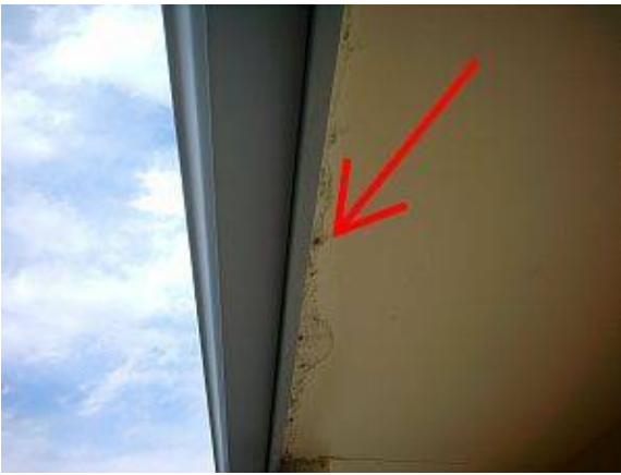
Photo 11 minor deterioration of soffit on back side
