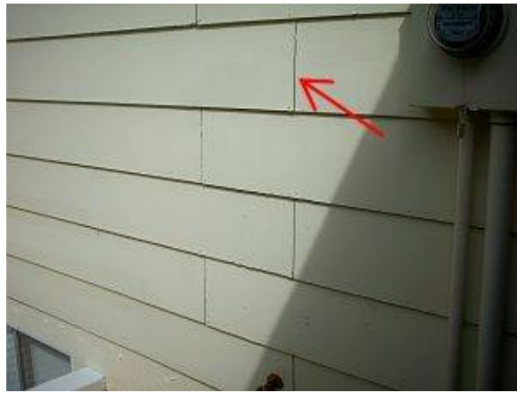
Photo 6 gaps between siding pieces
