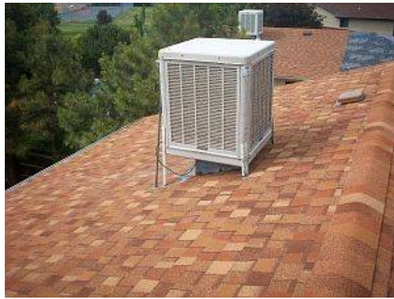
Photo 12 rooftop evaporative cooler
