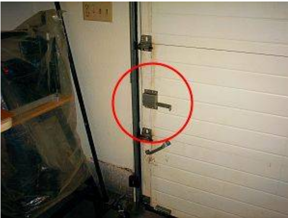
Photo 13 lock not disabled on garage door
