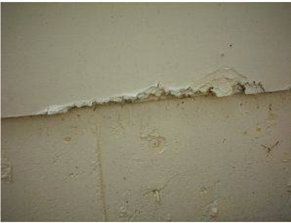
Photo 5 deterioration at lower edge of siding
