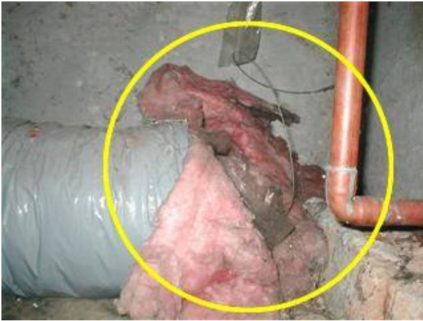
Photo 49 Broken duct in crawl space.
