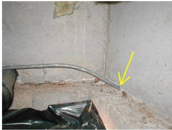
Photo 48 Abandoned wiring (for hot tub?) in crawl space.
