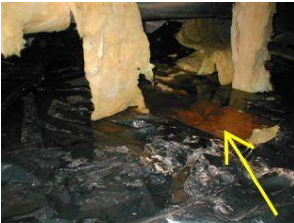
Photo 54 Standing water in crawl space.
