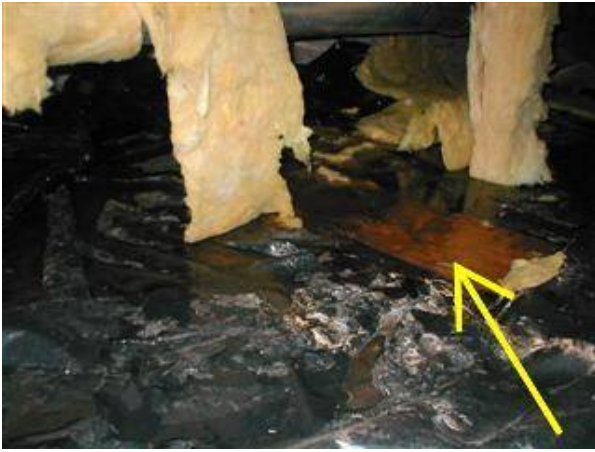
Photo 54 Standing water in crawl space.
