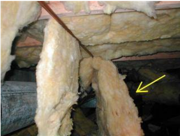
Photo 56 Fallen down under-floor insulation in crawl space.
