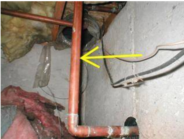
Photo 51 Main service water supply pipe in crawl space.
