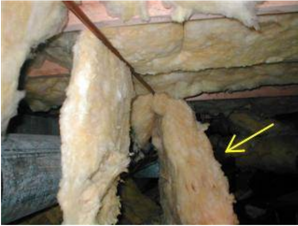
Photo 56 Fallen down under-floor insulation in crawl space.
