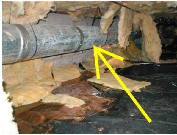
Photo 55 Ductwork insulation lying in water in crawl space.
