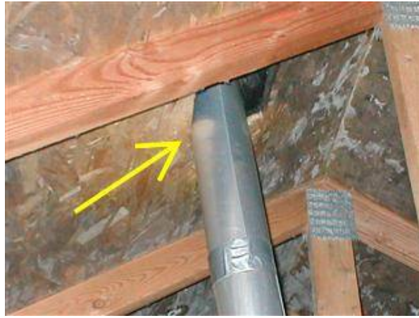
Photo 26 Exhaust fan duct blocking roof vent. Should have a dedicated vent cap.
