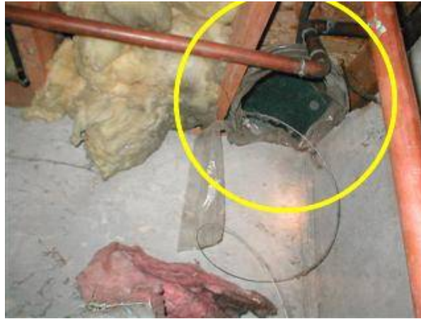
Photo 50 Other end of broken duct.
