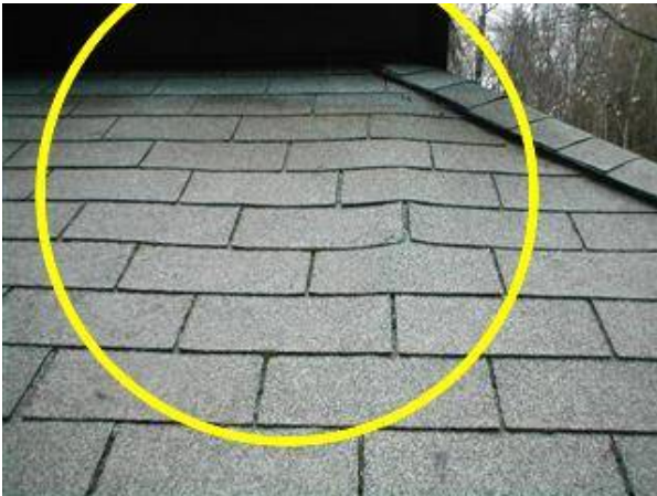
Photo 7 Uneven roof surface above front door.
