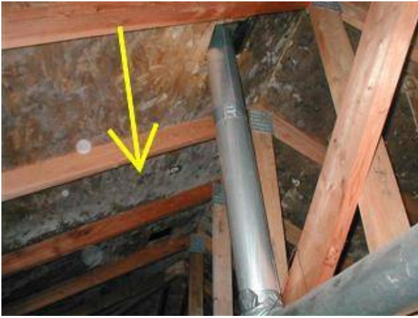
Photo 23 Discolored roof sheathing.
