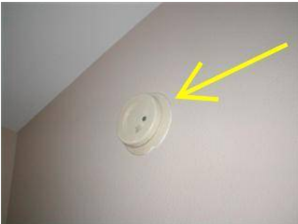
Photo 19 Possible older smoke detector.
