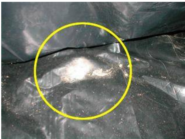
Photo 53 Dead mouse between layers of vapor barrier in crawl space.
