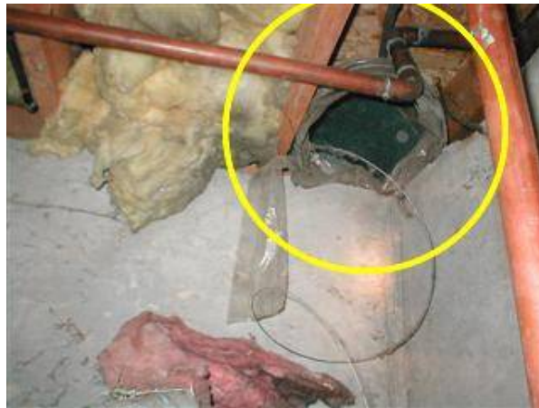
Photo 50 Other end of broken duct.
