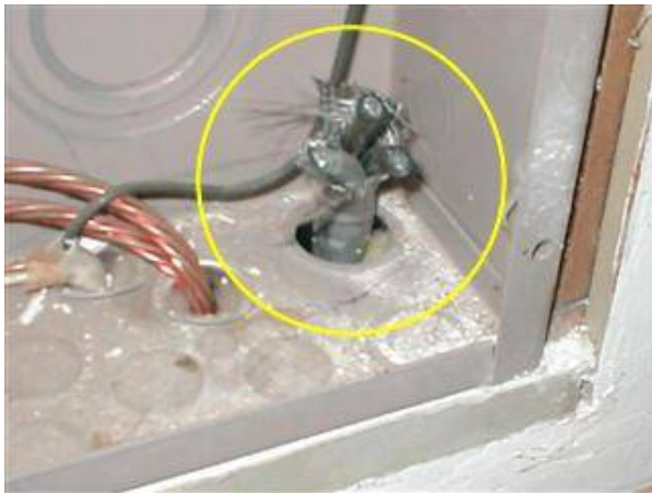
Photo 14 Abandoned wiring with no bushing in main service panel.
