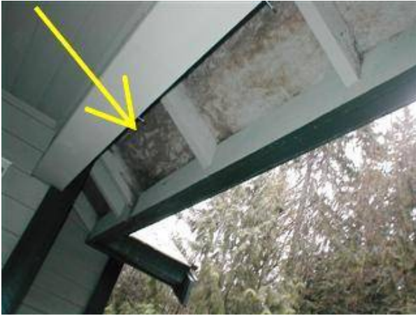
Photo 38 Dark colored roof sheathing over front porch.
