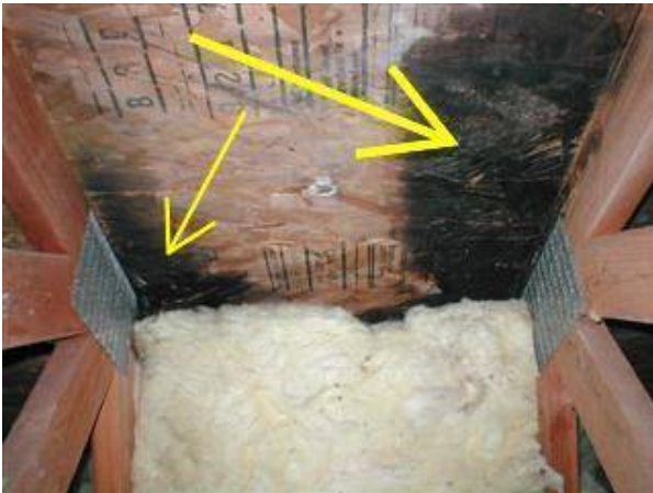
Photo 21 Blackened roof sheathing by skylight chase.
