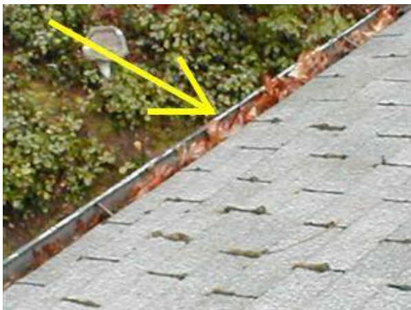
Photo 8 Debris in gutters.
