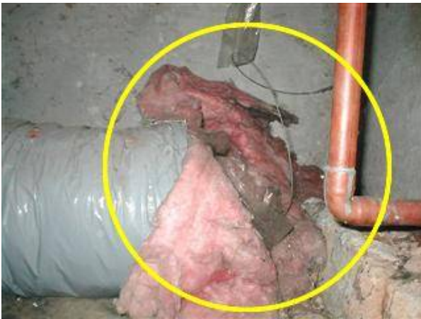
Photo 49 Broken duct in crawl space.
