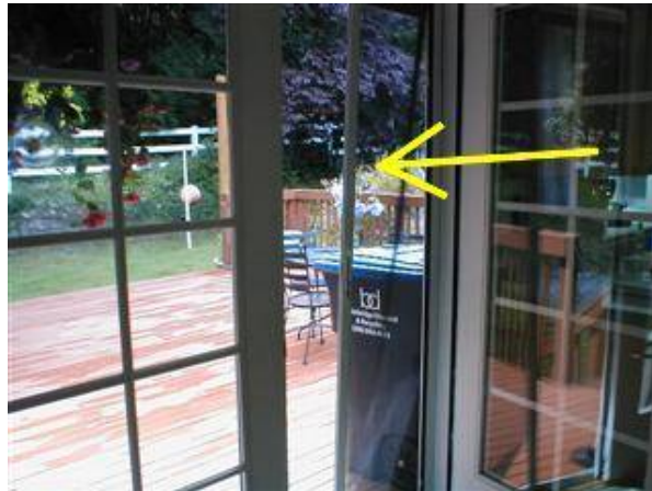
Photo 33 Screen door at kitchen difficult to open and close.
