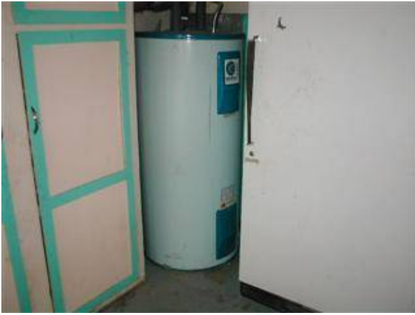
Photo 19 Older water heater.
