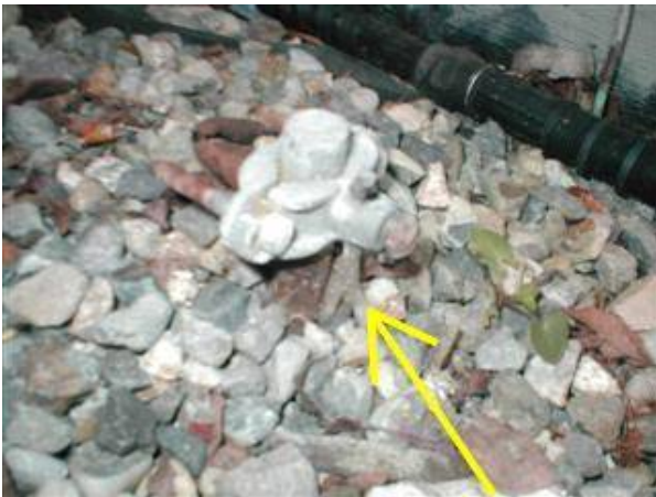
Photo 9 Loose clamp on ground rod.
