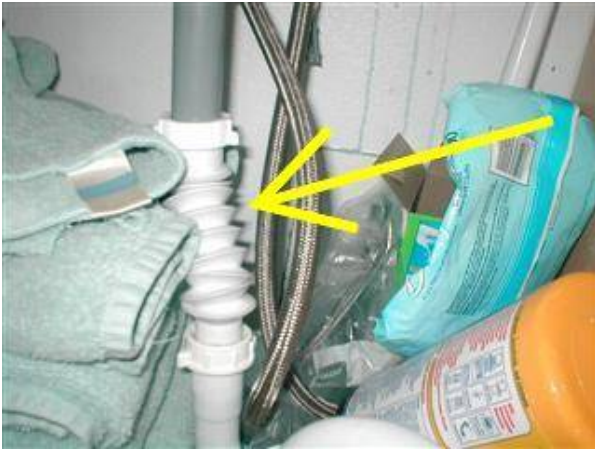
Photo 35 Flex pipe used for upstairs bathroom sink drain.
