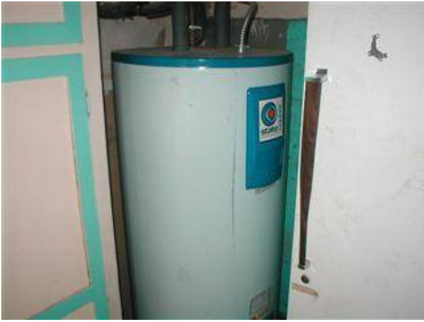
Photo 18 No seismic straps.
