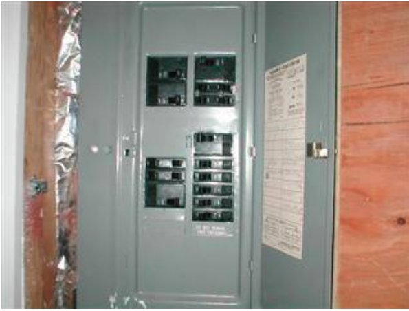
Photo 24 Split bus main service panel.
