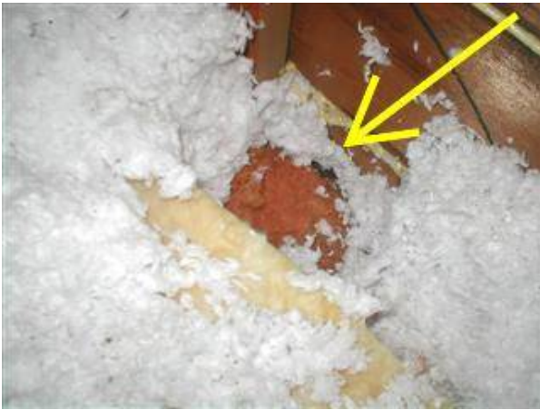
Photo 30 Silva wool insulation below newer loose fill fiberglass insulation in attic.
