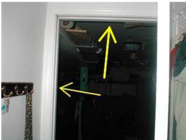
Photo 12 Weatherstrip missing from garage-house door.
