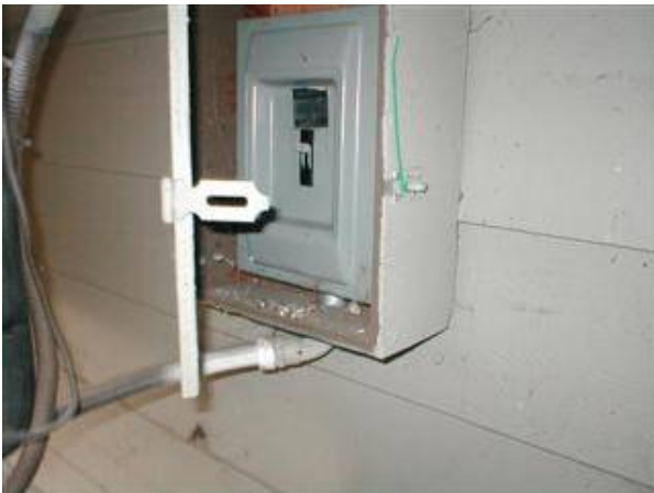
Photo 5 Wooden enclosure prohibited removal of subpanel cover.
