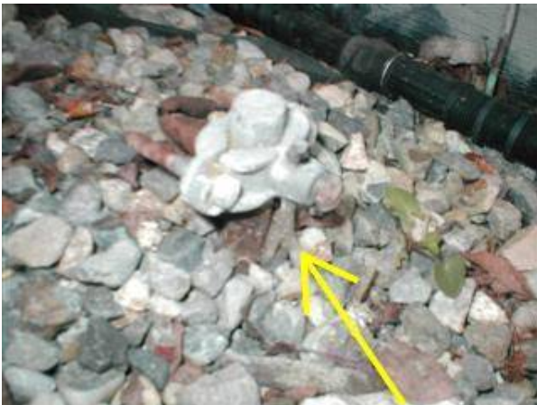
Photo 9 Loose clamp on ground rod.
