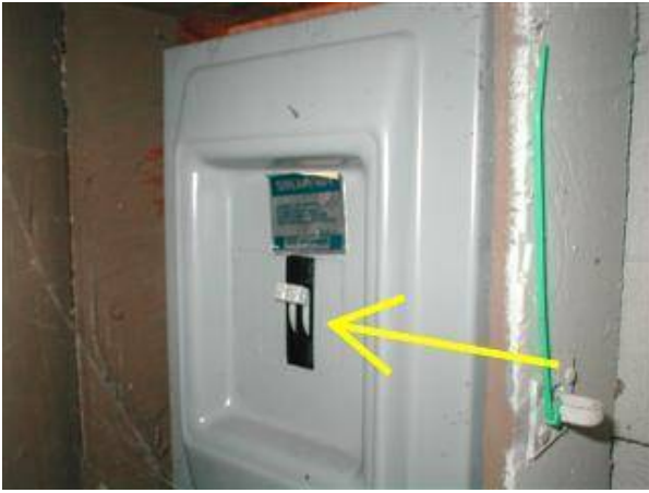
Photo 4 Zinsco breakers used at heat pump disconnect panel.
