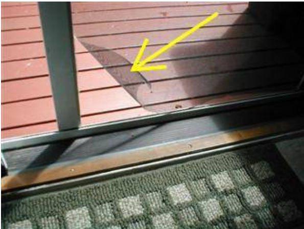
Photo 32 Torn screen in kitchen entry door.
