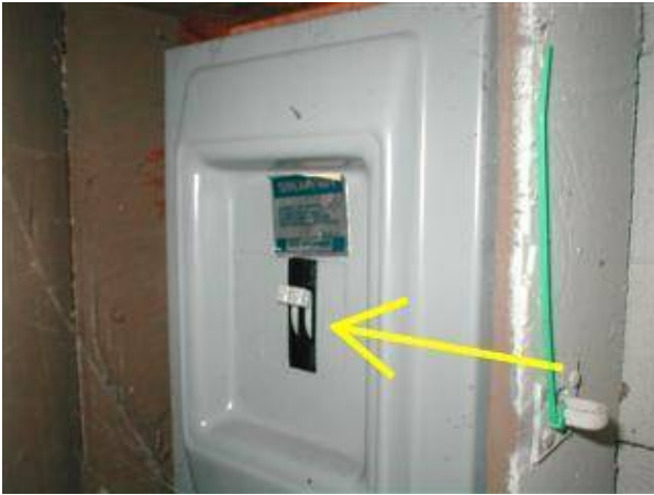
Photo 4 Zinsco breakers used at heat pump disconnect panel.
