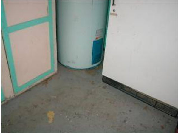
Photo 20 No 18" pedestal for water heater located in garage.
