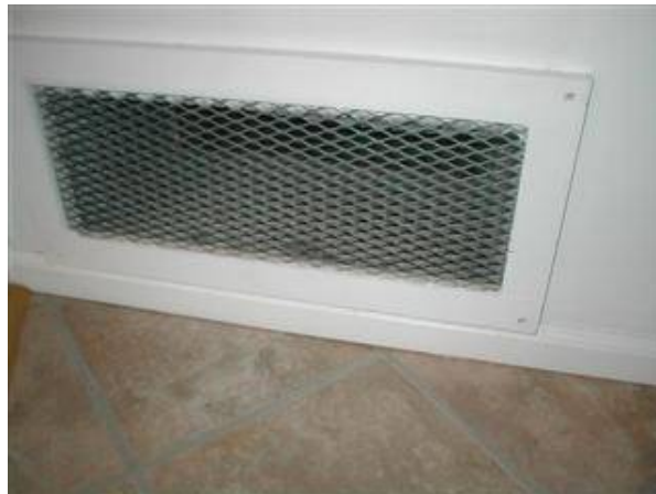
Photo 28 No filter at downstairs return air grill.
