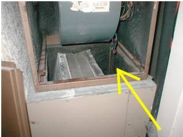
Photo 26 No filter at base of furnace.
