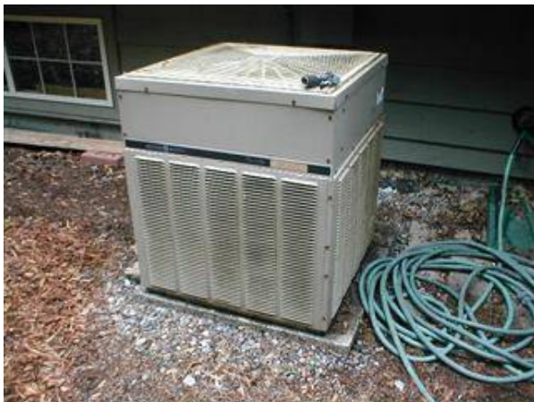
Photo 6 Older heat pump.
