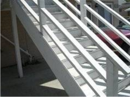
Photo 8 Gaps in rail should not exceed 4-1/8" for child safety.
