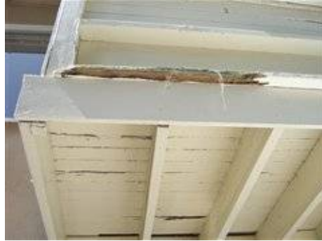
Photo 13 Consult termite report.
