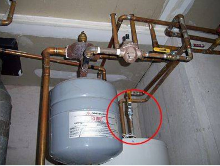
Photo 11 Leak at one or more shut off valves.
