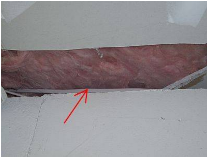
Photo 8 Exposed fiberglass insulation.
