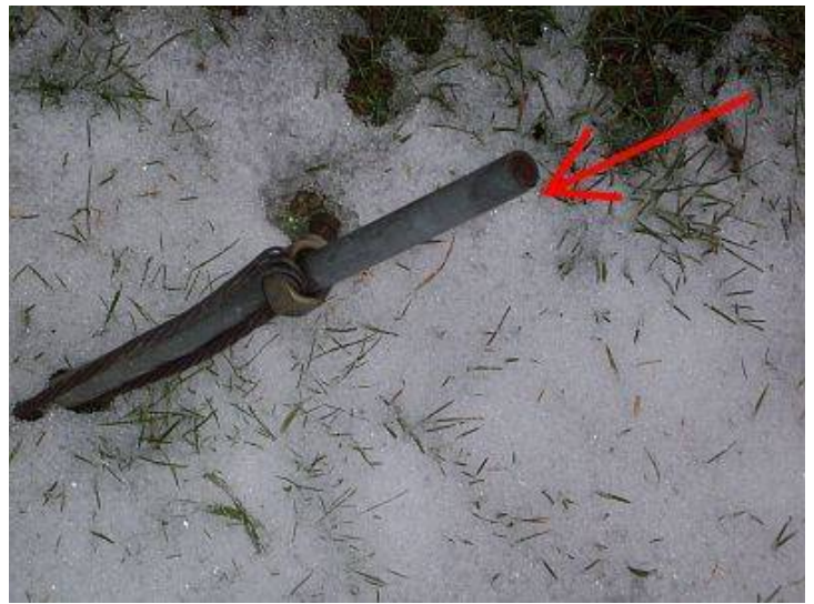
Photo 6 Exposed grounding rod extending ~ 1 ft out of ground.
