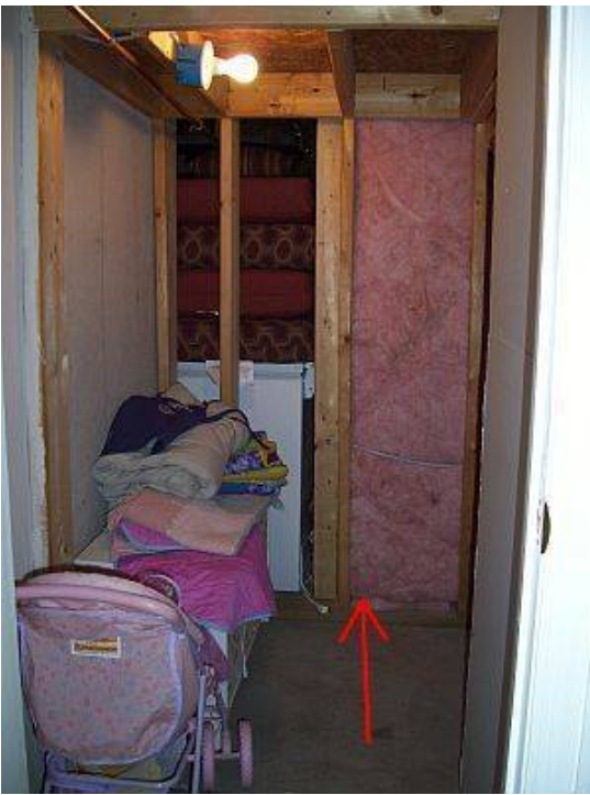
Photo 14 Exposed fiberglass insulation in storage area beneath stairs. Walls and ceiling unfinished.
