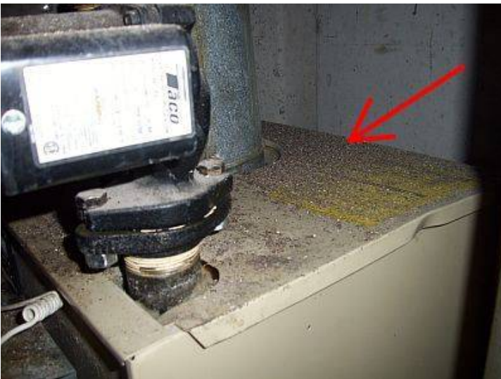
Photo 10 Ashes found from opening in ceiling; fireplace above it on first floor.
