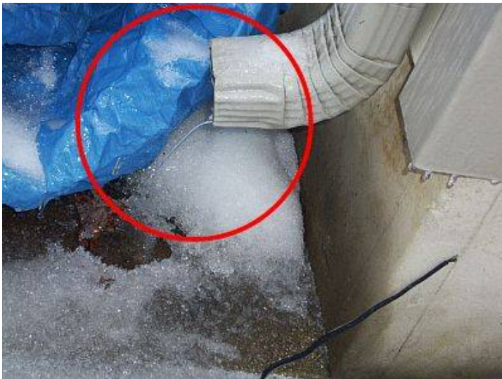
Photo 3 Missing downspout extension.
